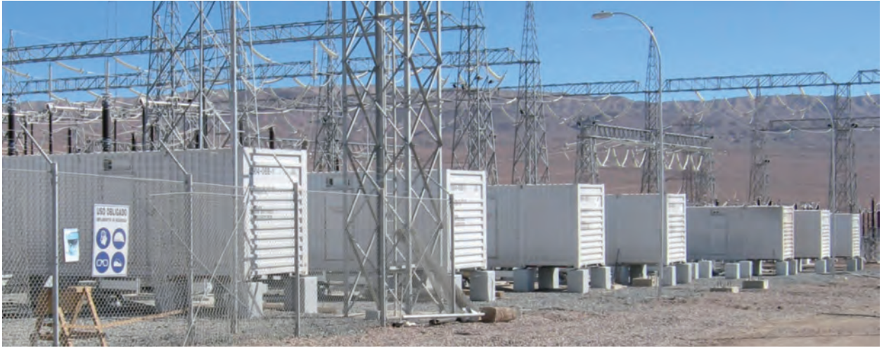
Figure 3-3 – Li-ion battery supplying up to 12 MW of power at Los Andes substation in Chile (A123, 2009)
