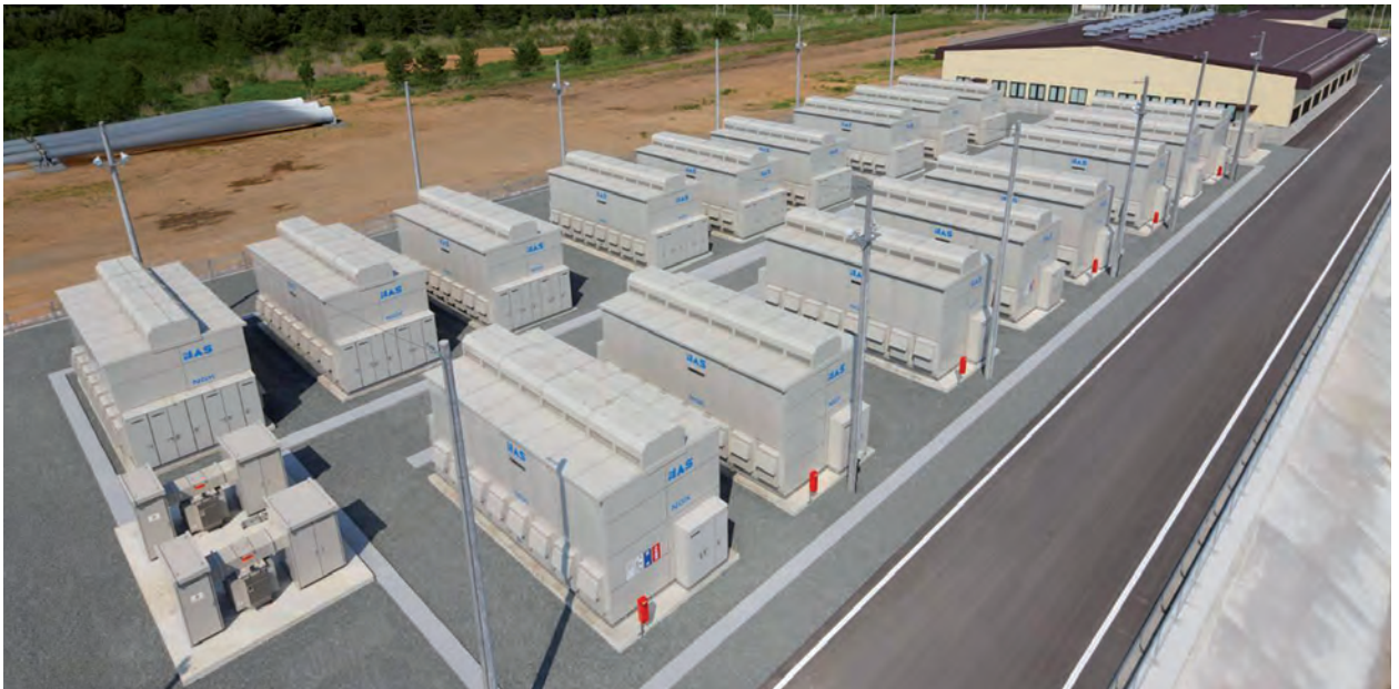
Figure 3-10 – NaS battery units – 34 MW (Japan Wind Development Co.)
